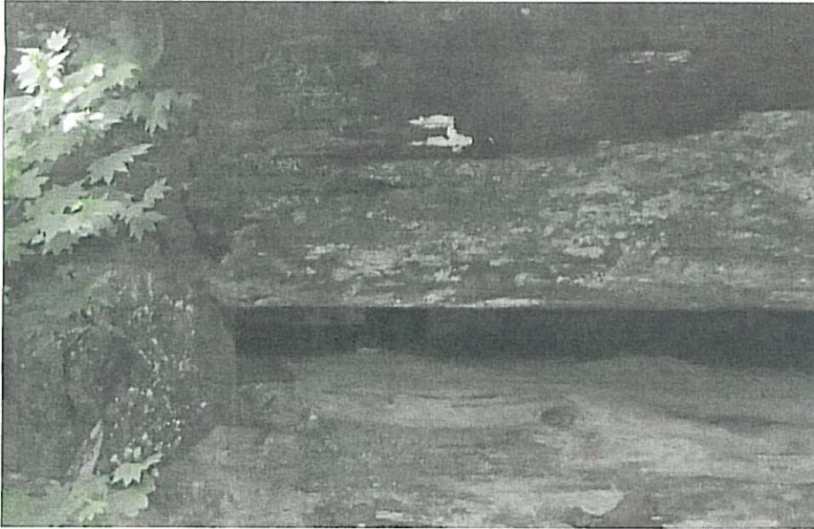
CK-2261 Pier Span Downstream Crack
